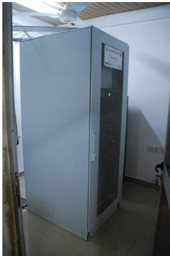
Photo 18: GMA, Central Processing Equipment in Tema ACC in an air conditioned room.
