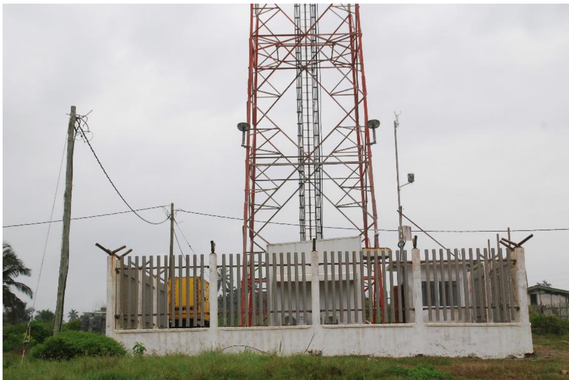
Photo 10: Remote Sensor Site (RSS): fence, tower, generator (yellow), air conditioned server room (in front of the tower) and office (on the right side of the tower) in Winneba
