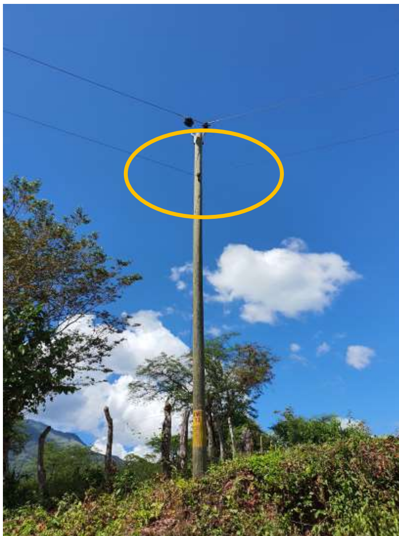
Figure 7: Spigot insulator failure
