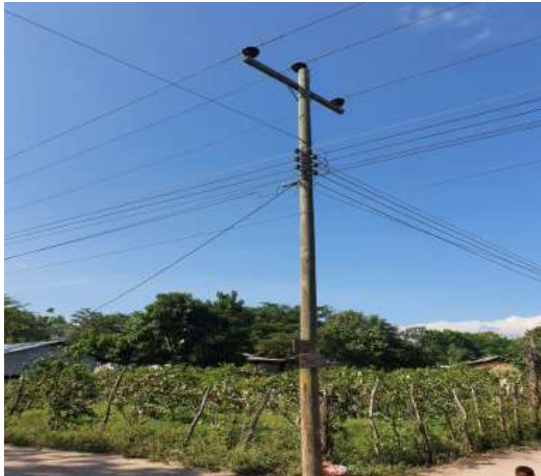
Figure 1: Primary structure, 3 phases, 34.5 kV.
