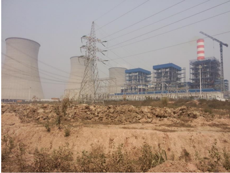
Figure Error! No text of specified style in document.-1 Hongsa Power Plant
